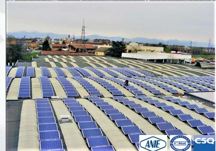
424,32 kWp Rooftop PV System installed in Italy - Tribiano (MI)
